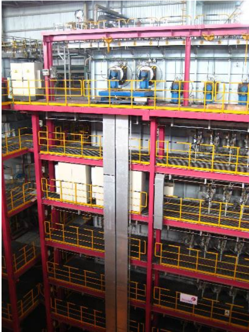
Partial view of a vertical furnace in a continuous annealing line with steering roll expansion joints in the upper area. Image: ©Frenzelit GmbH
